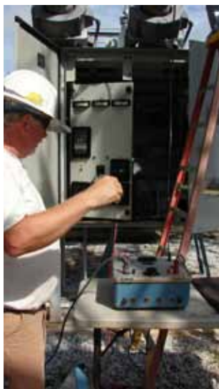
Breaker Contact Resistance
