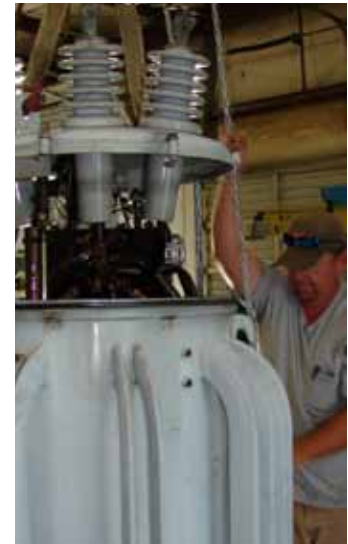
Shop Disassembly of a Regulator
