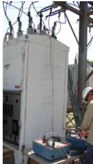
Hi Pot Testing a Vacuum Circuit Breaker
