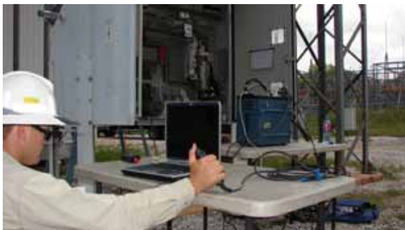
High Tension Breaker Timing
